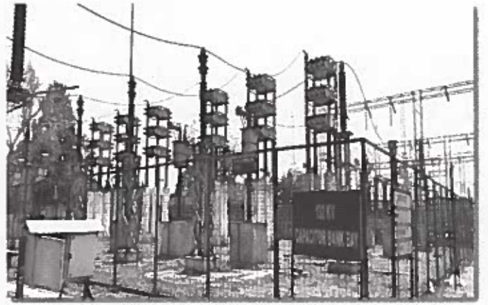
Figure 1: 132kV Capacitor Bank at 220kV Sub-station Sarojini Nagar
