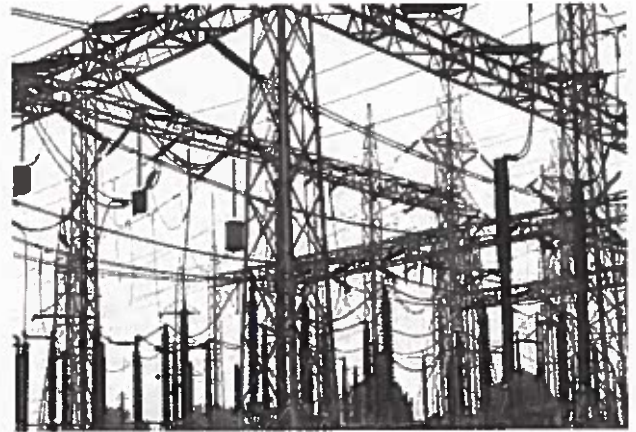
Figure 3: Strengthened 220kV Bus Bar (Single moose to twin moose conductor)
